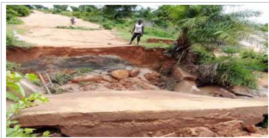
Figure 5.2: Collapsed portion of the bridge linking Maajin Kaji and other communities in Lavun LGA, Niger state due to heavy downpour Photo: Sode Mohammed/Radio Nigeria.
