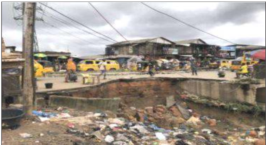
Figure 4.5: Ikotun/Ejigbo road in Lagos Collapses After a heavy downpour
