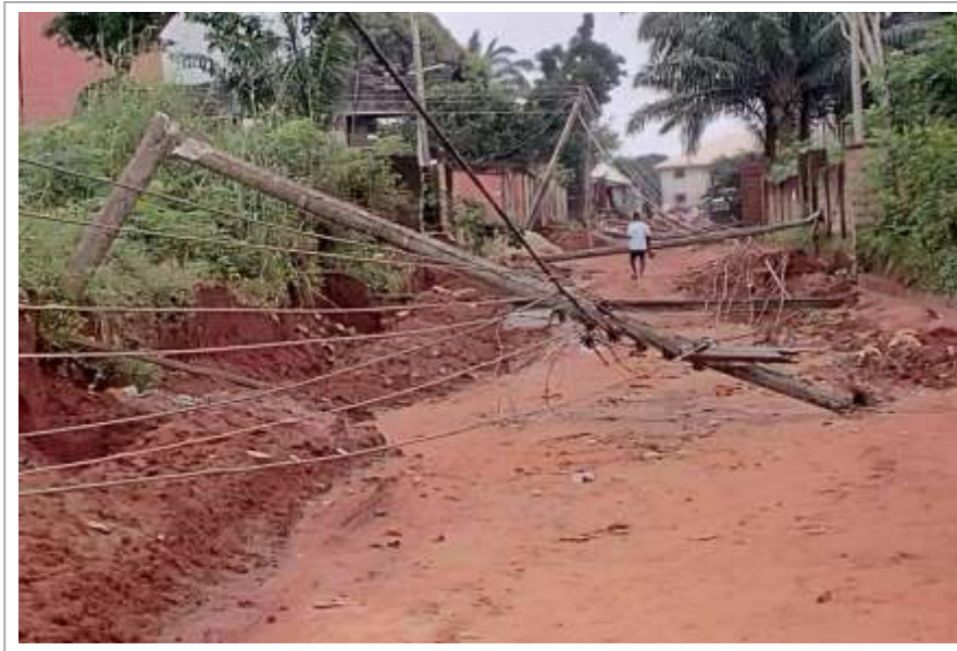
Figure 5.3: Fallen poles at Adabebe village in Amawbia Community Awka South Local Government Area 14
