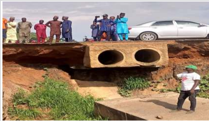
Figure 4.17: Erosion washes away bridges, threatens houses in Bauchi (Source: Premium Times, August 28 2023)
