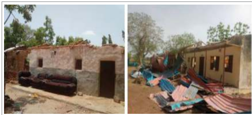
Figure 4.14: Damaged shelters in Bauchi wind storms (Source: IOM UN Migration)
