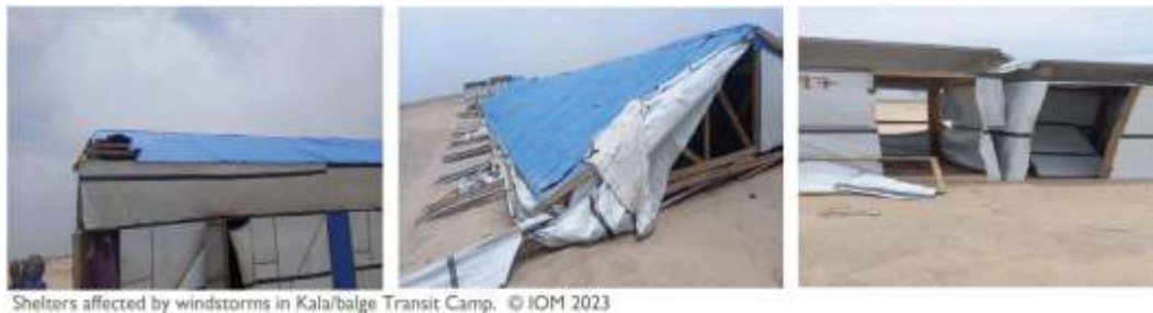
Shelters affected by windstorms in Kala/balge Transit Camp. © IOM 2023
