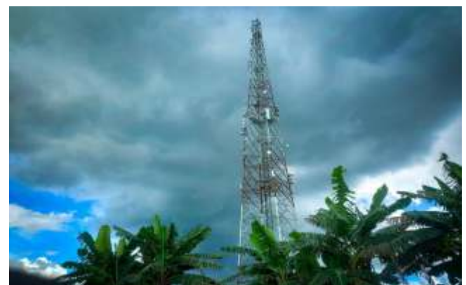
Figure 44: Mobile Network Tower
