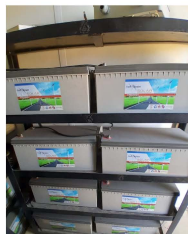
Figure 1.5: Set of 200Ah Batteries in Kano
