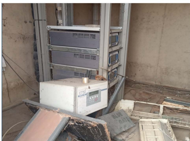
D. Figure 3.2 a-d: Damaged sensors and Air conditioning system in the portal cabin at Maiduguri Air quality Station damaged by severe storm since 2016
