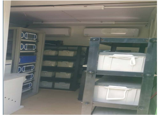
Figure 7.2: The analyzers of Abuja Air Quality stations (Not functioning)
