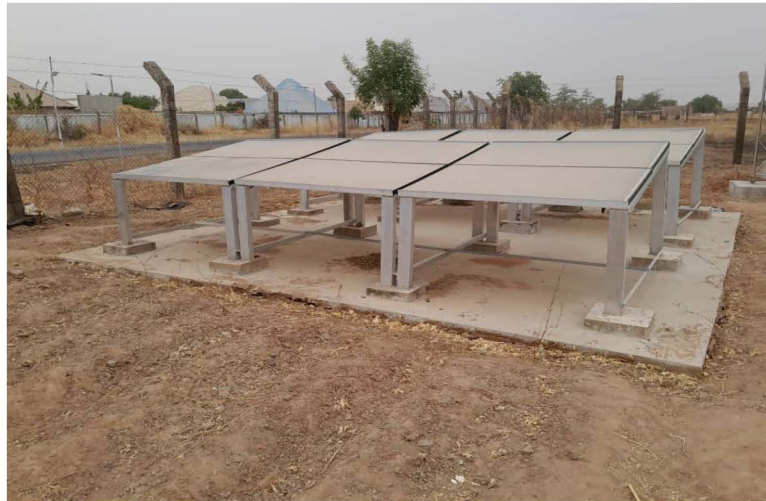
Figure 4.2: The Solar Panel installed (Not yet functioning)
