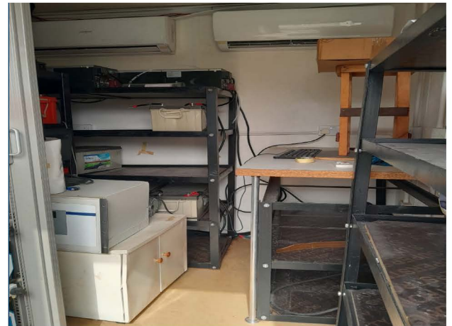
Figure 6.4: Interior of the cabin showing the Air Conditioning systems (Not functioning)
