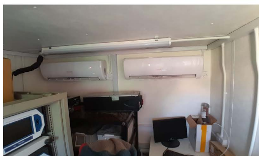
Figure 1.4: Inside cabin of Kano air quality stations showing ACs, and the Analyzers left in the station uninstalled since 2017
