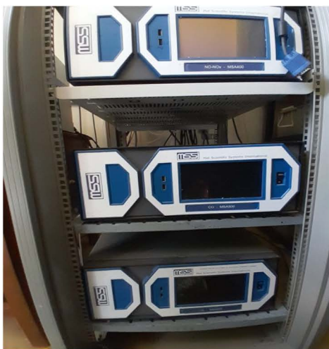
Figure 1. 2a: Kano Gas pollutant Analyzers
