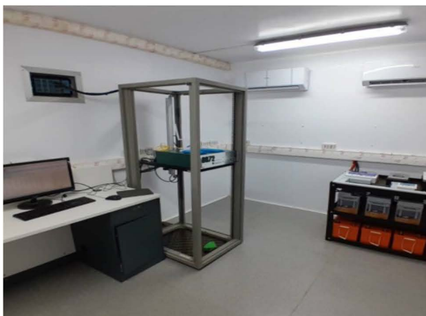
Figure 2.2 Interior of Porta Cabin showing Batteries, Inverter, Data logger and display unit in Sokoto
