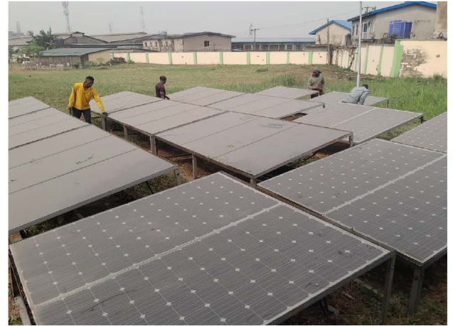
Figure 6.2: Solar panel installed in Lagos Air quality station
